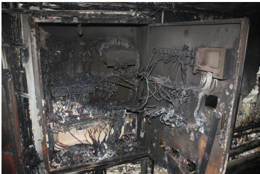
Fig. 1 A fire accident in switchboard 1)
